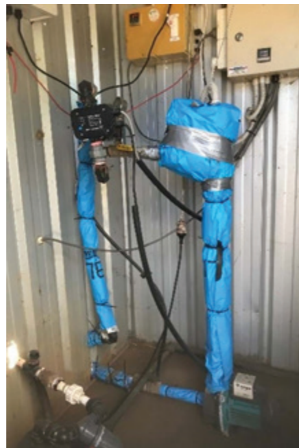
The simplest fix is to insulate your heating head pipes and if possible, the distribution pipes . . .
